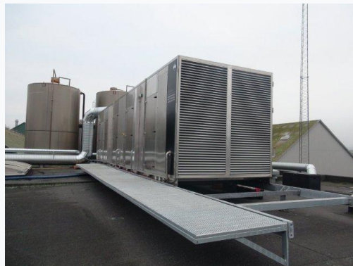
GPAO system at water treatment plant, Aarhus Denmark
