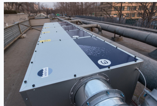
GPAO system at the Royal Danish Embassy in Beijing
