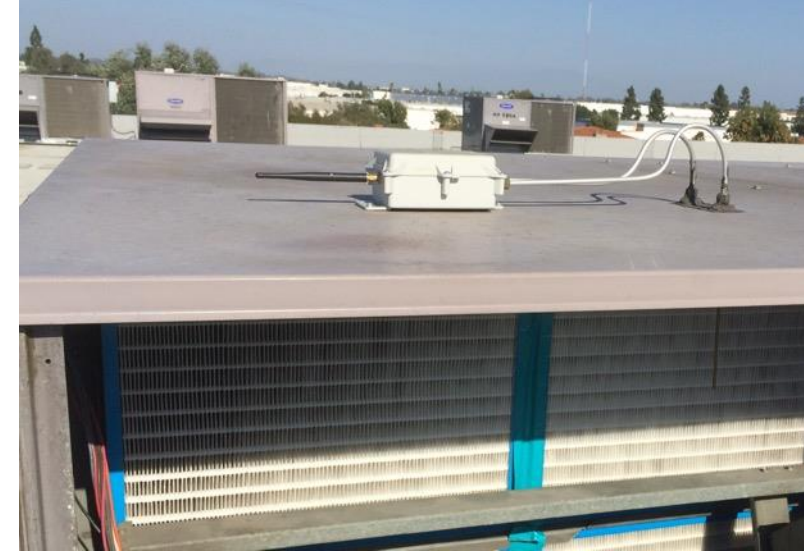
Wireless differential pressure sensor installed on roof air handler
