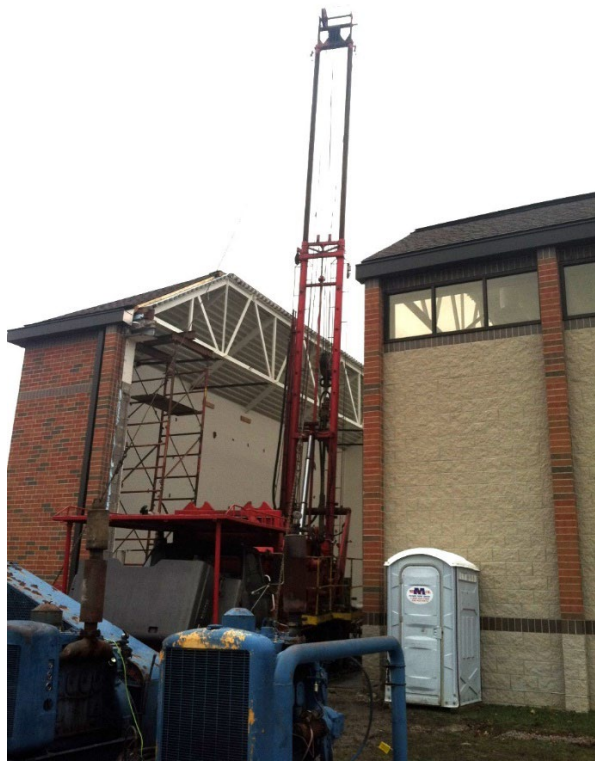
School gymnasium built over a plugged well, which began leaking. Photo courtesy of Ohio Dept. of Natural Resources, Division of Oil & Gas Resources Management.
