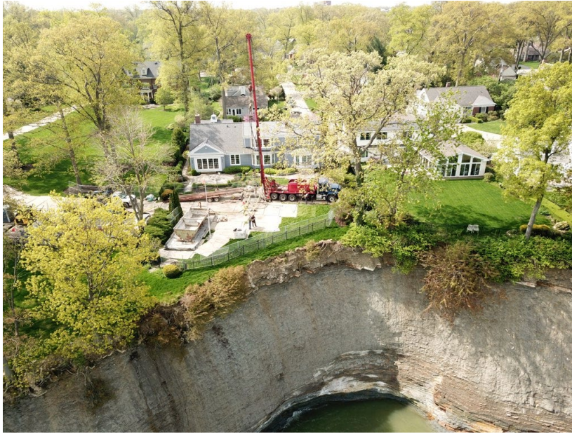
Orphan well plugged above an approximate 50 to 60 foot high wall along the Lake Erie shoreline, which is being undercut by the lake. Photos courtesy of Ohio Dept. of Natural Resources, Division of Oil & Gas Resources Management.
