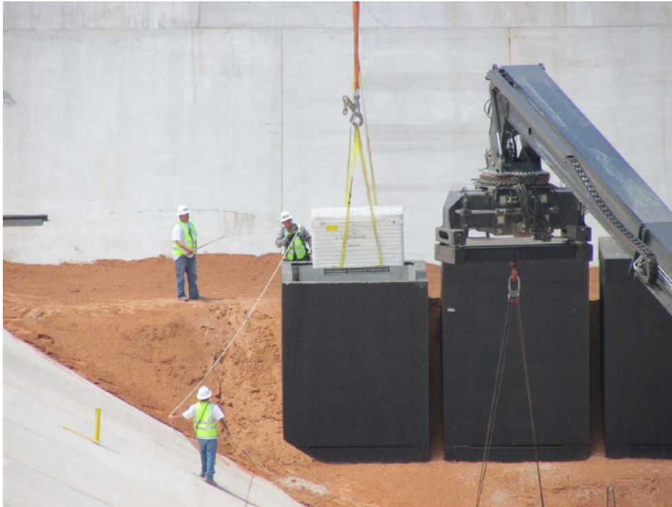
Rectangular MCC holds four B-25 DOT shipping containers
