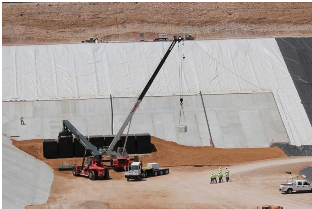
Figure H-3 Rectangular MCCs inside a Disposal Cell with Components of Multi-Barrier Liner are Visible in the Background
