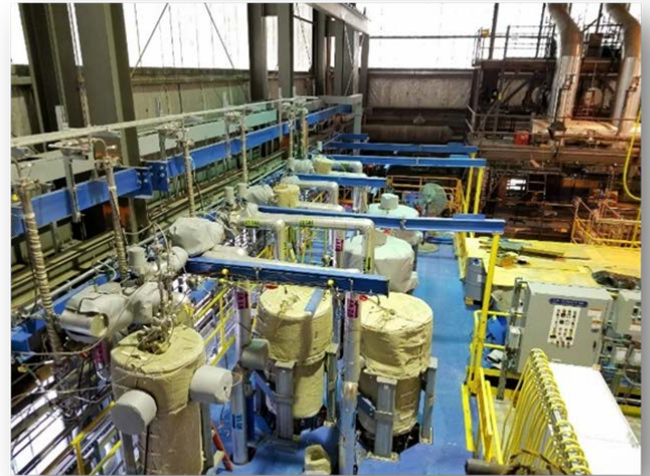
METL Facility, Argonne National Laboratory
