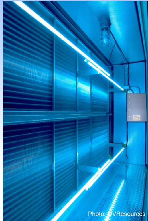
Leaving Side of Evaporator Coil
