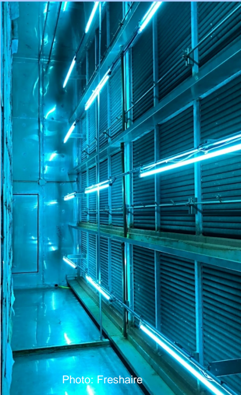
Entering Side of Evaporator Coil
