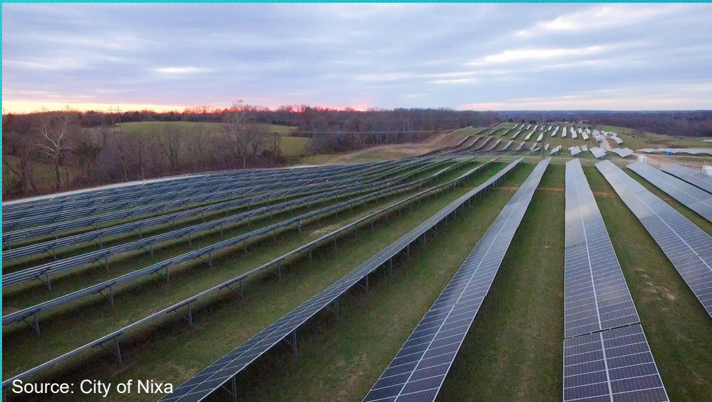
SWPA customer solar farm in Missouri
