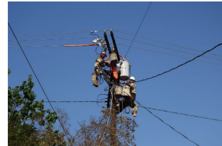
New Distribution Voltage Conversion →
