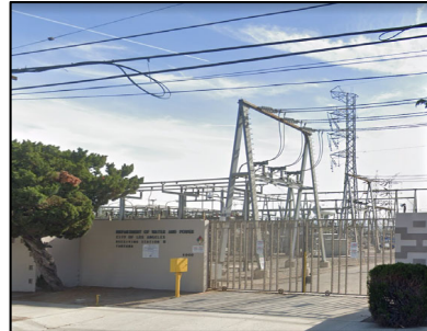
New Distributing Stations
