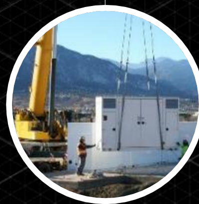
Ft. Carson, CO Battery Energy Storage System
