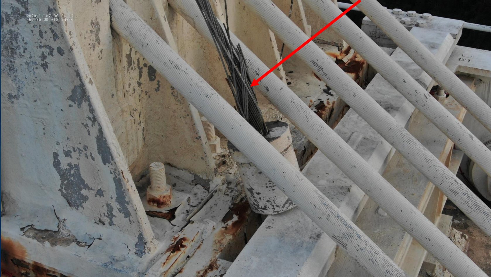
Failed main cable
