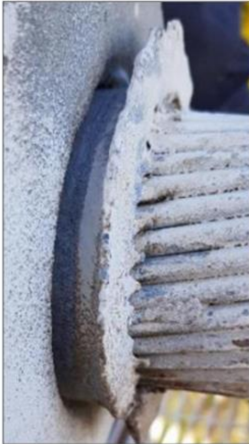
Socket M8N_T exhibited 3/4" cable slip.
