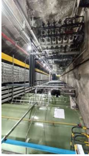
Ultra Purity Water system
