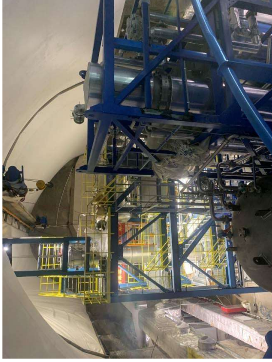
Underground LS hall
