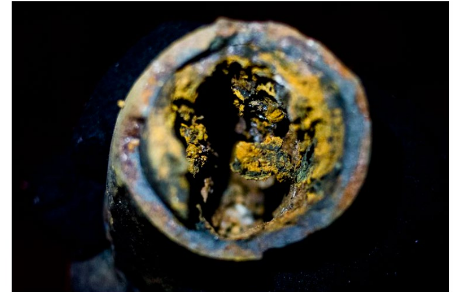
One of the first lead pipes that was removed from Veronica Kelly's home shows the extent of the corrosion the harder Flint River water has had on Feb. 22, 2016 at her home on the city's north side. (Jake May | MLive.com)
