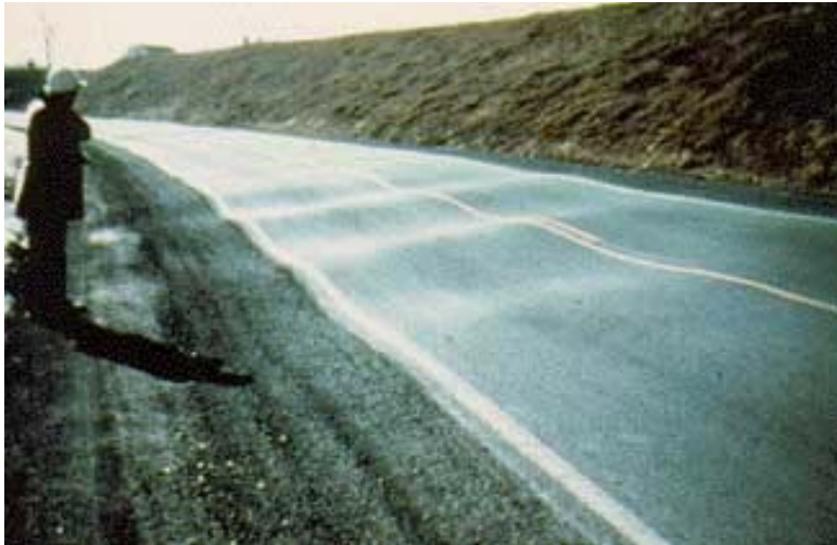
Pavement Damage Due to Frost Heave
