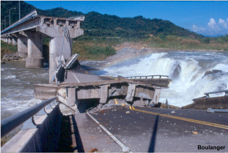
Surface Fault Rupture – 1999 Chi-Chi earthquake in Taiwan
