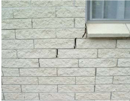
Settlement-Induced Masonry Cracking
