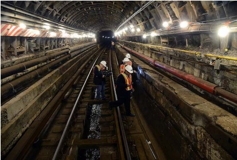
Montague Tunnel One Year after Hurricane Sandy
