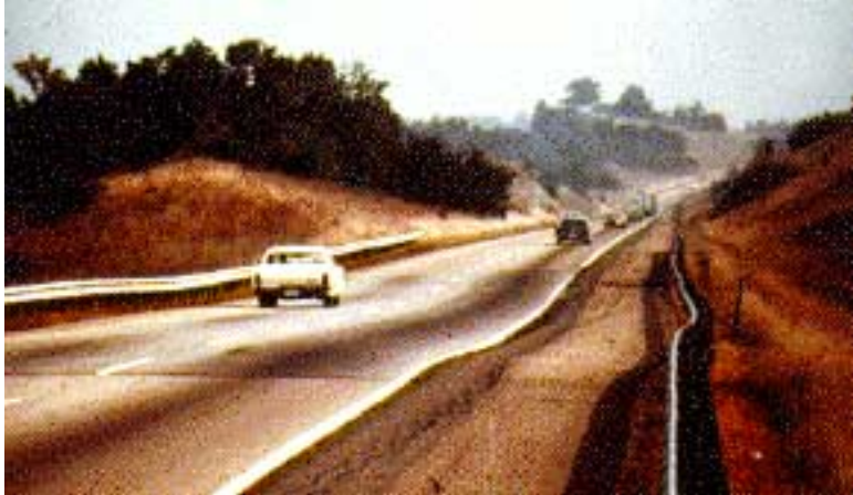
Pavement Damage Due to Expansive Soils
