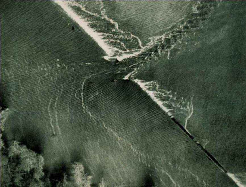
Catastrophic levee overtopping and failure
