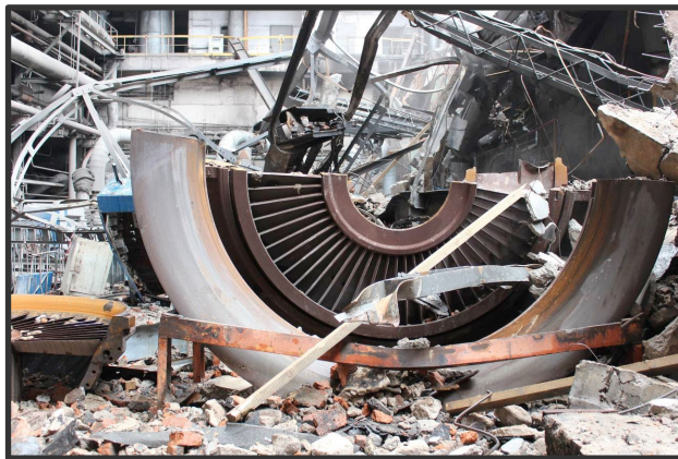
DTEK images of destruction caused by russian attacks against DTEK power station in March 2024
