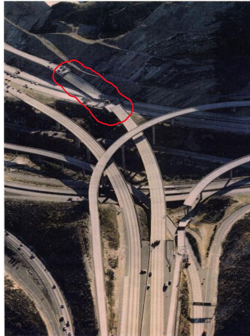
Route 14/Interstate 5 Interchange Collapsed Connectors 53-1964F & 53-1960F
