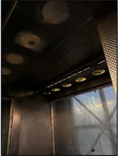
Damaged elevator resulting from misuse by individuals engaging in substance use at the Slauson BRT Station. Source: David Cooper
