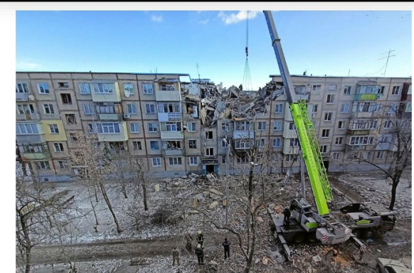
Rescuers remove debris from a residential building damaged by an airstrike, as Russia's attack on Ukraine continues, in Kharkiv, Ukraine March 15, 2022. REUTERS/Vitalii Hnidy
