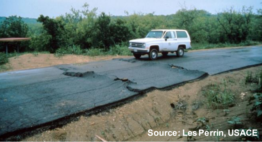
Heaving on Joe Pool Lake Road, Grand Prairie, Texas
