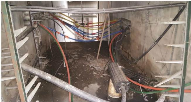
Figure 5-5. Details of the interior of the vault contents within a picture.
