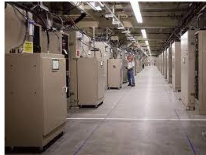
Capacitor banks ( \sim 400 MJ)
