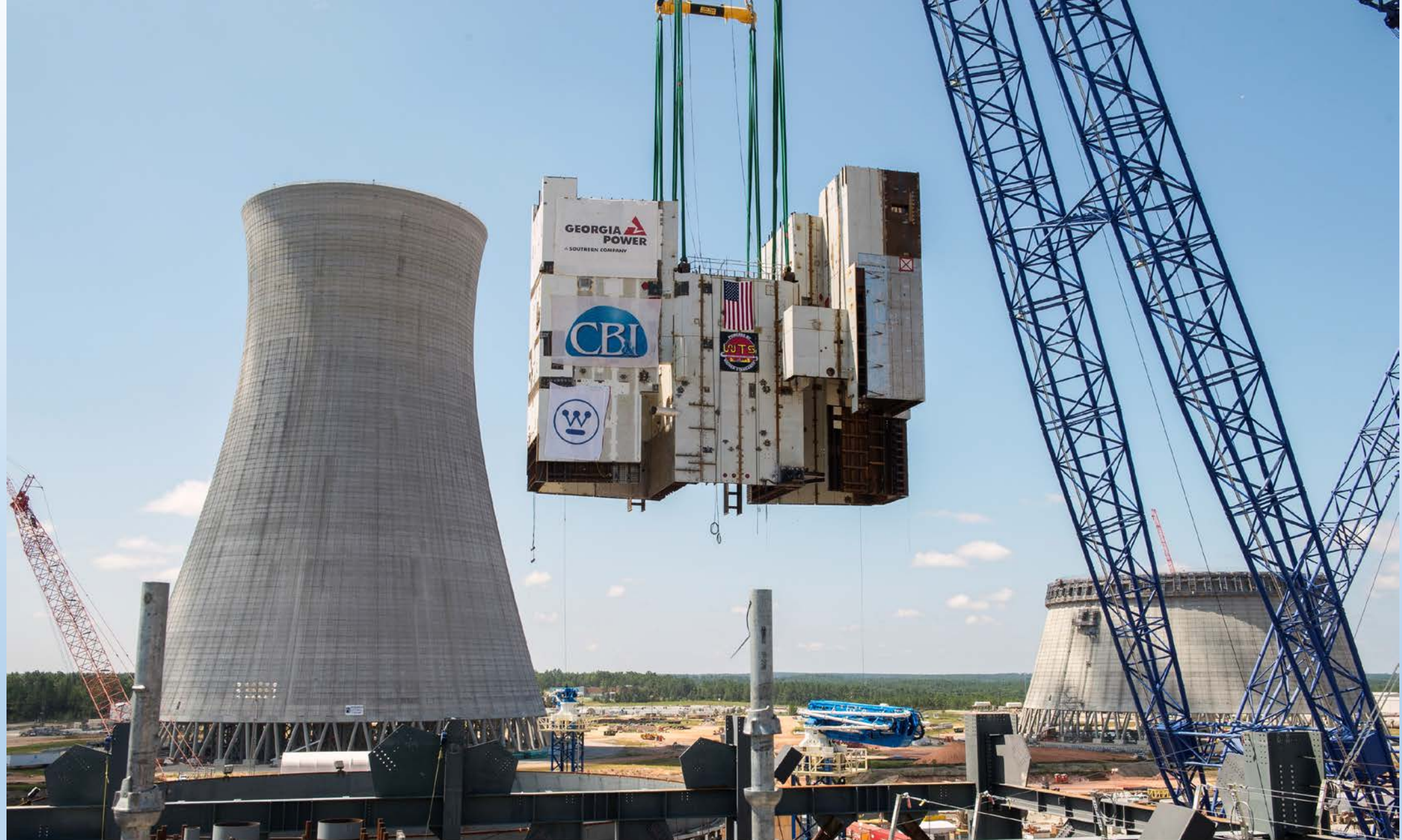
Lifting over 1,200 tons, the heavy lift derrick places the CA01 module inside the Vogtle Unit 3 containment vessel.
