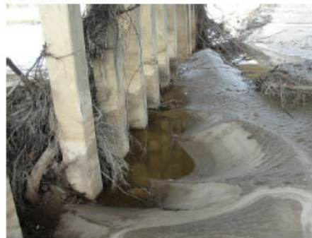
Figure 7-2. Scour Damage at Bent (Padgett et al. 2020b)
